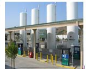
NG and LNG station, US
